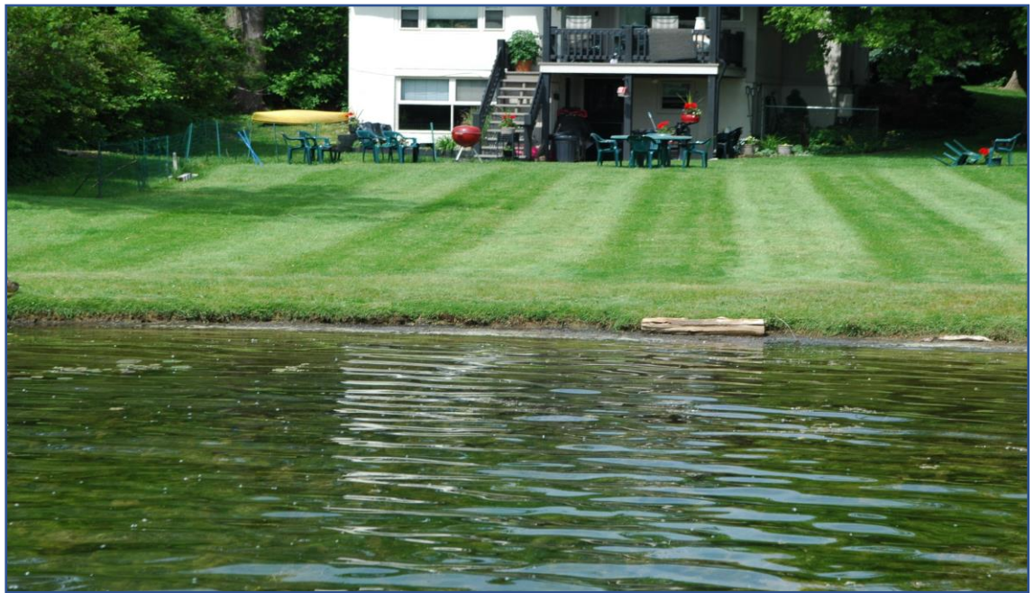
Figure 55. An example of poor shoreline management with no vegetation buffer present. ©RLS
